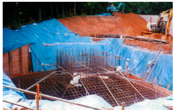
Fig. 11. Father Costantino Ruggeri and Luigi Leoni, St. Francis Xavier church, Yamaguchi, 1993-98; construction of the foundation for the two towers.
