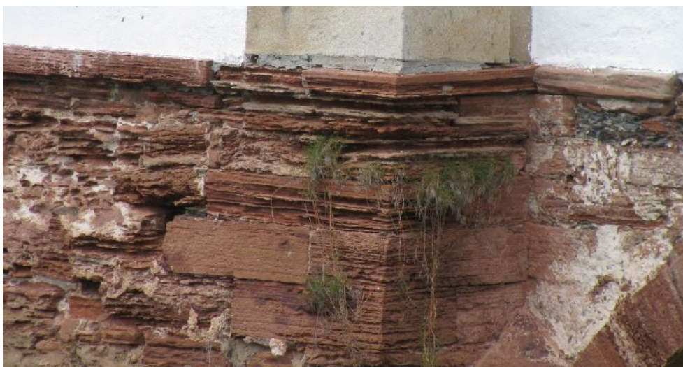
Fig. 3. Examples of sedimentary stones intense erosion that might have impact on stone reusability in a bridge in Ilhavo (Central Portugal).
