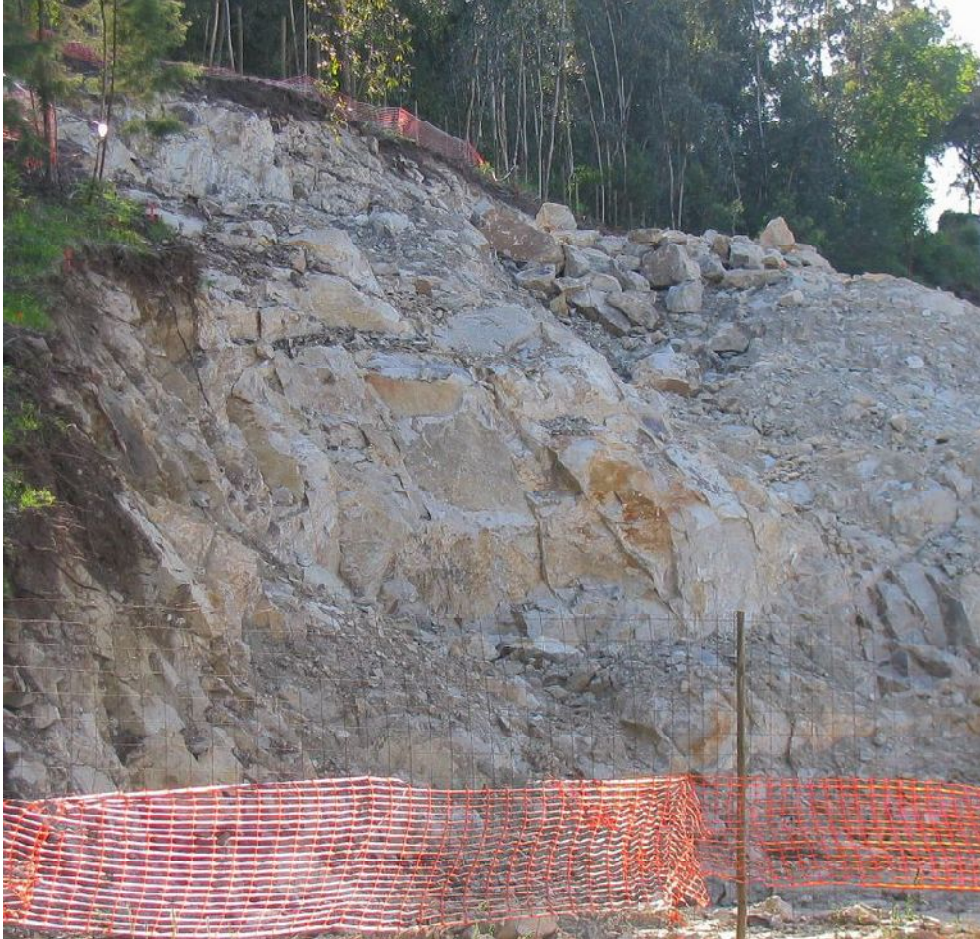
Fig.2. Road excavation in granite rock massif producing rock debris (Braga, Northern Portugal).
